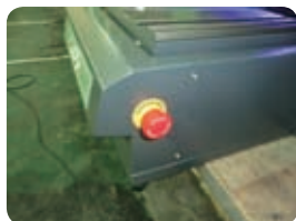
Emergency stop device system
