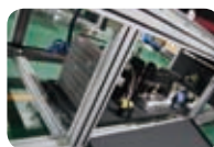
Water cooling system for UV lamp
